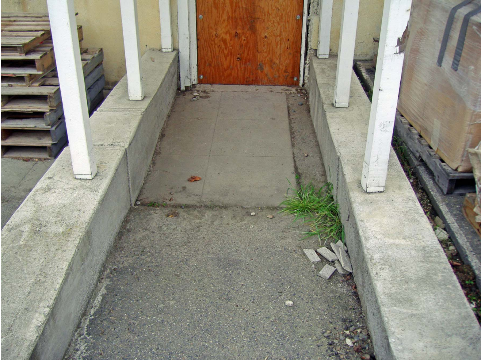
Detail of Concrete Work in Area of Doorway on North Elevation (facing South).
