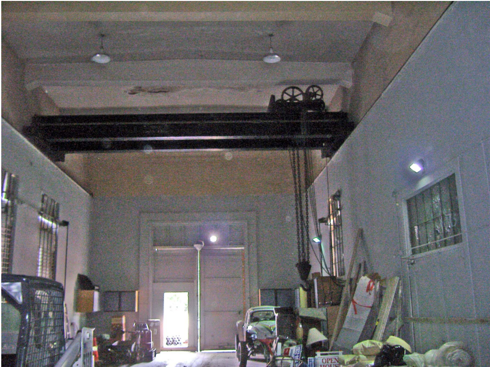
Overview of Interior of SD G & E Building with Crane (facing North).
