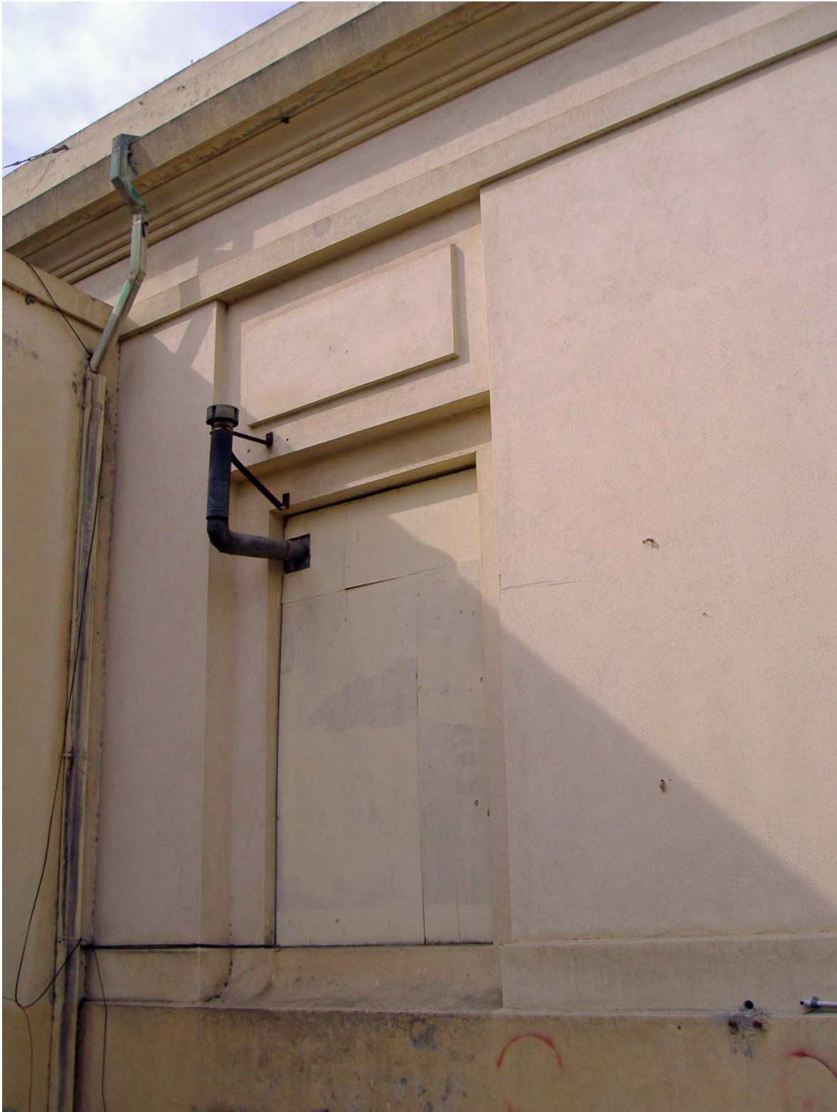
Detail of Covered Window on South Elevation of Western Portion fo SD G & E Building (facing West/Southwest).
