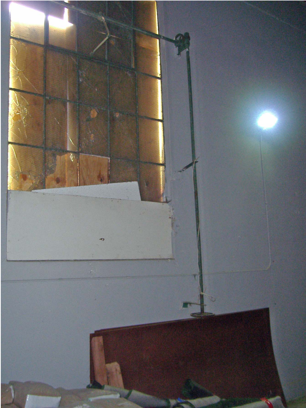
Example of Industrial Window with Crank-Handle Opener, East Elevation from Interior of Building (facing Southeast).
