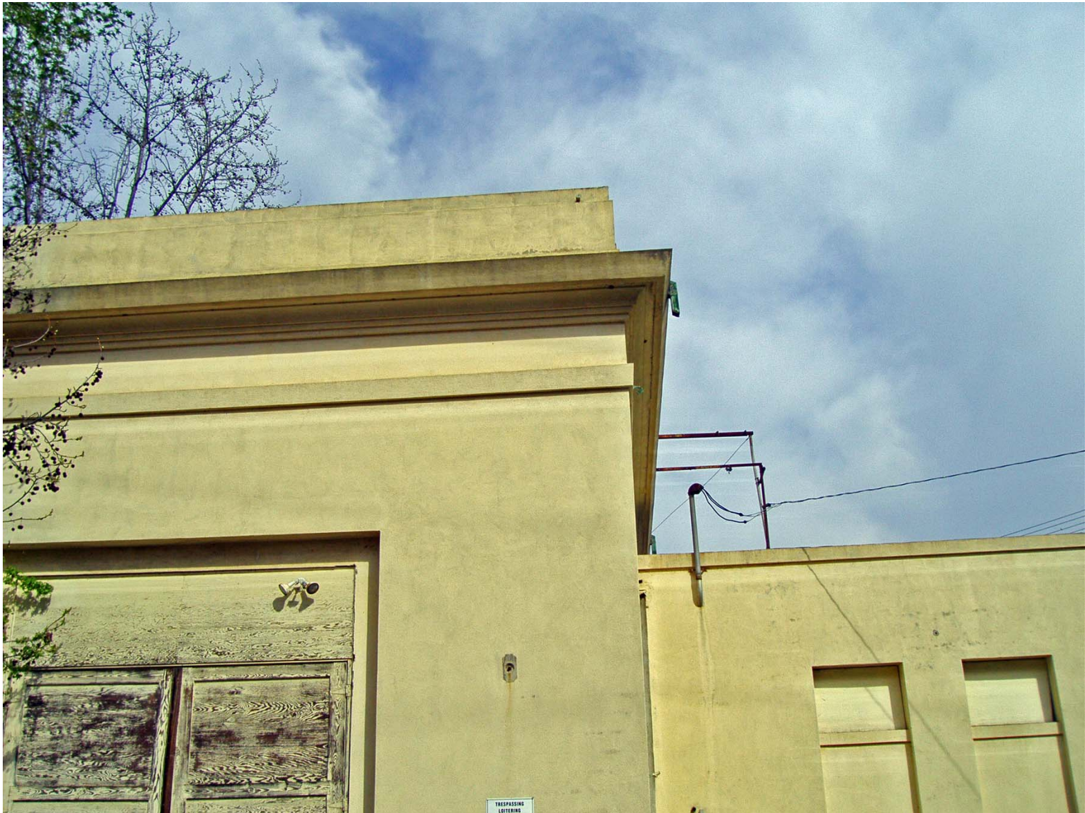
Detail of Roof Line on South Elevation fo SD G & E Building (facing North).
