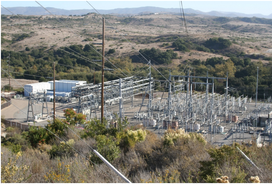
Photograph 11: View of developed area at the Talega substation.
