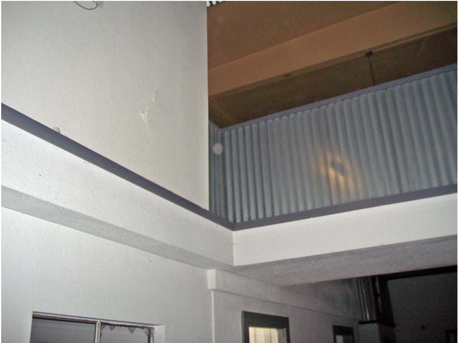
Railing Outside Second Story Offices of SD G & E Building (facing Southwest).
