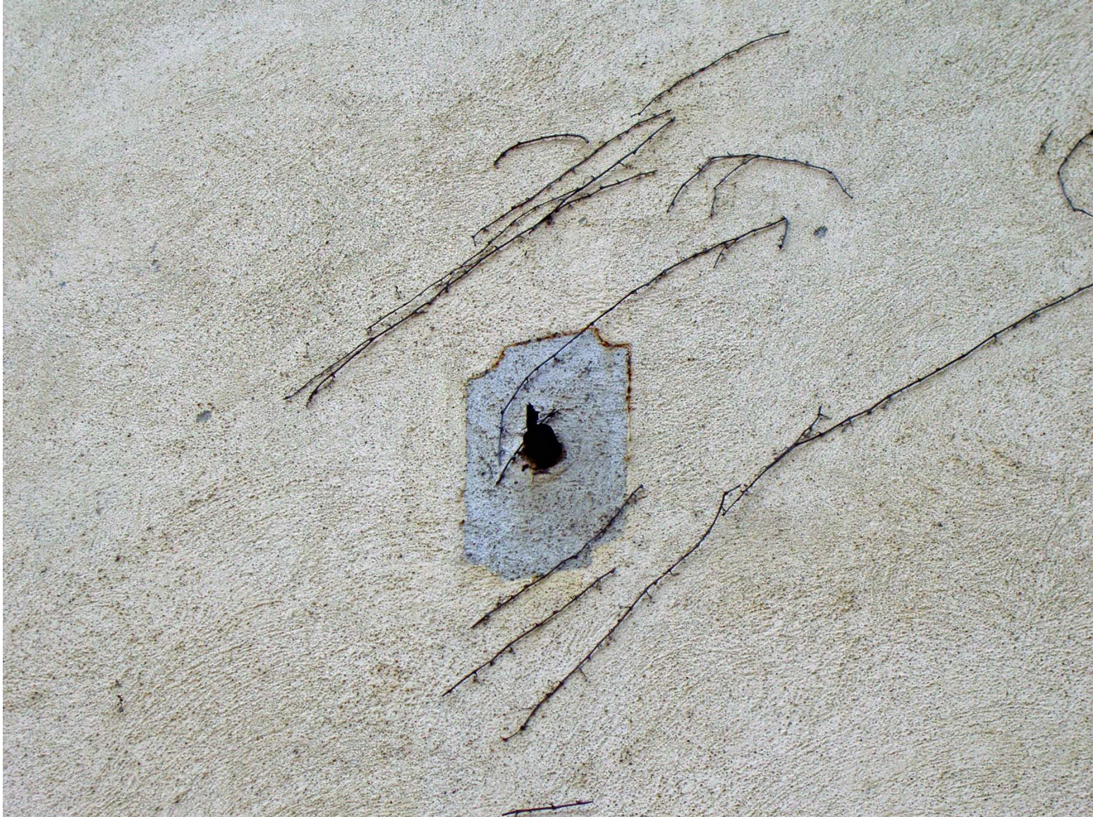
Detail of Scarring on North Elevation where Light Fixture was Removed (facing South),
