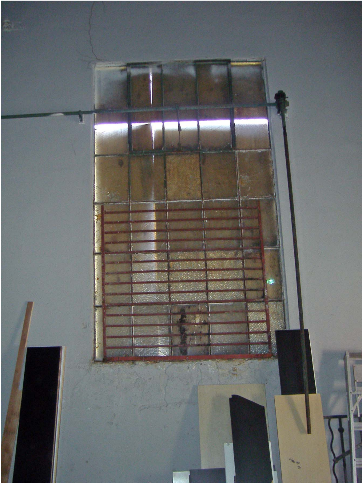
Dtrail of Fixed Industrial Windows within the SD G & E Buildings, San Juan Capistrano (facing West).
