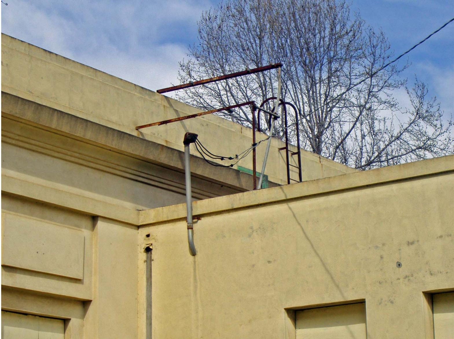
Utility Hook-ups and Roof Ladder on SD G & E Building (from South; facing Northwest).
