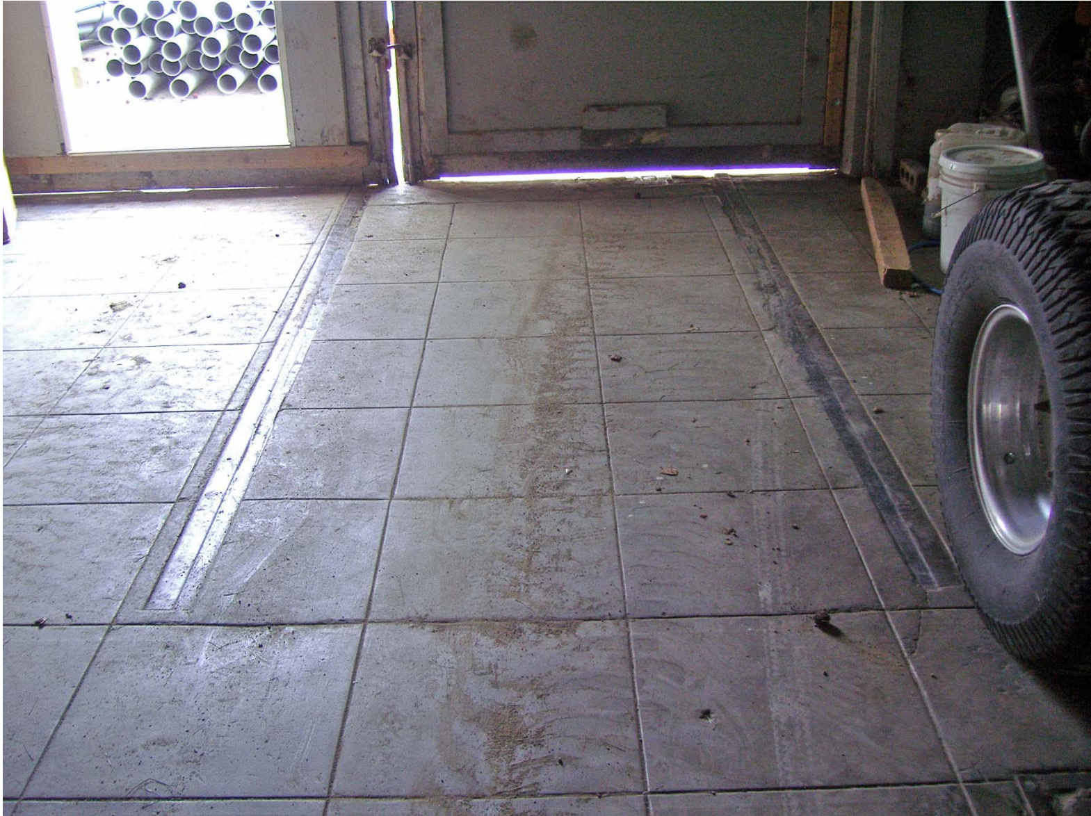
Detail fo Puoured Concrete Floor with Remnants of Rail Tracks (facing North).
