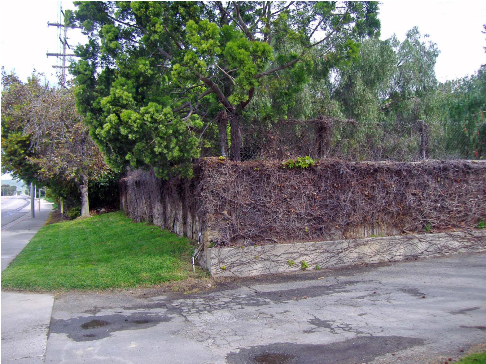
Overview of Wooden Fence on Concrete Sill to North of SD G & E Building (facing North/Northeast).
