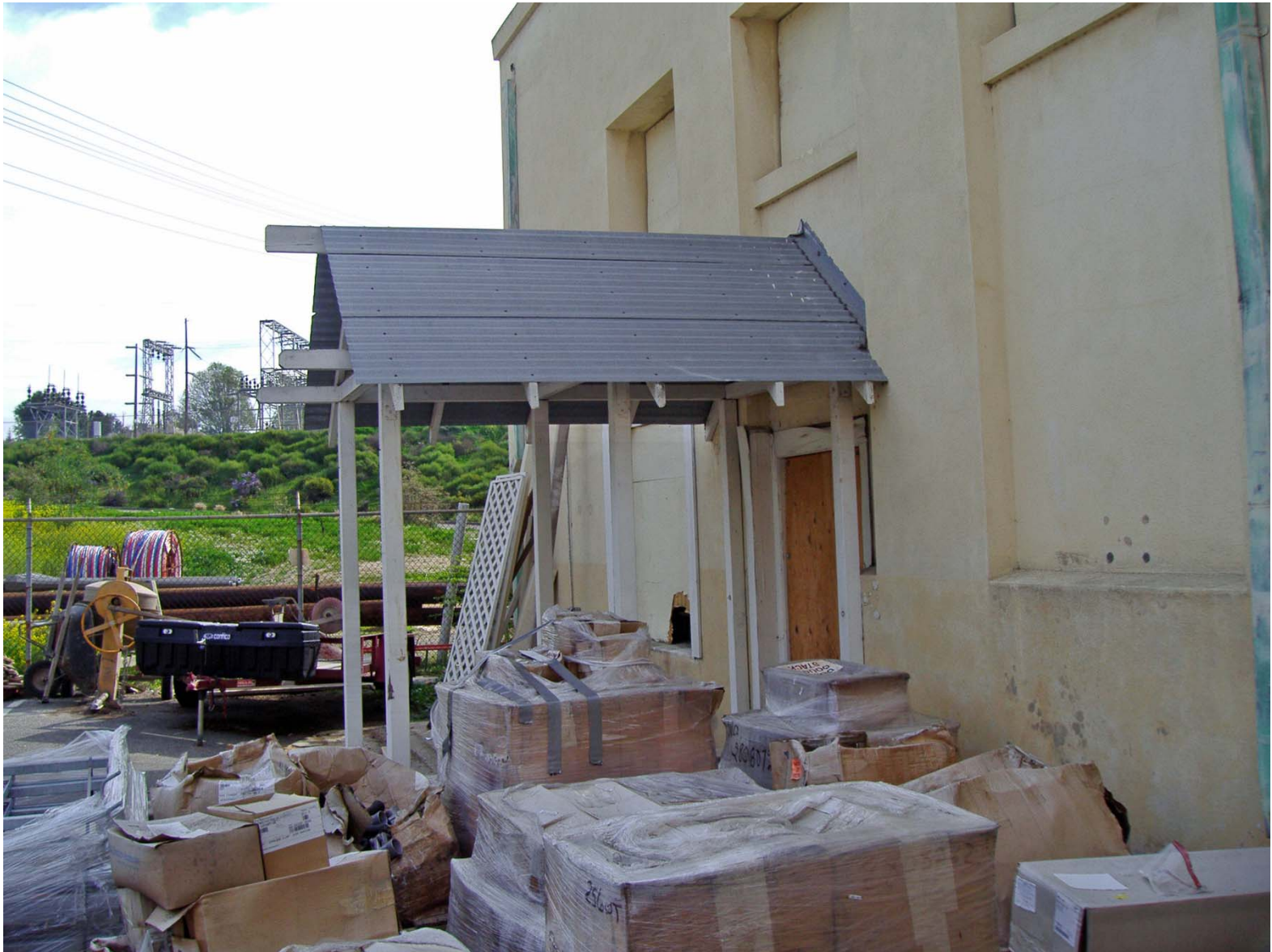
Overview of North Elevation with Added Covered Entry and Misc. Debris in Yard (facing Southeast).
