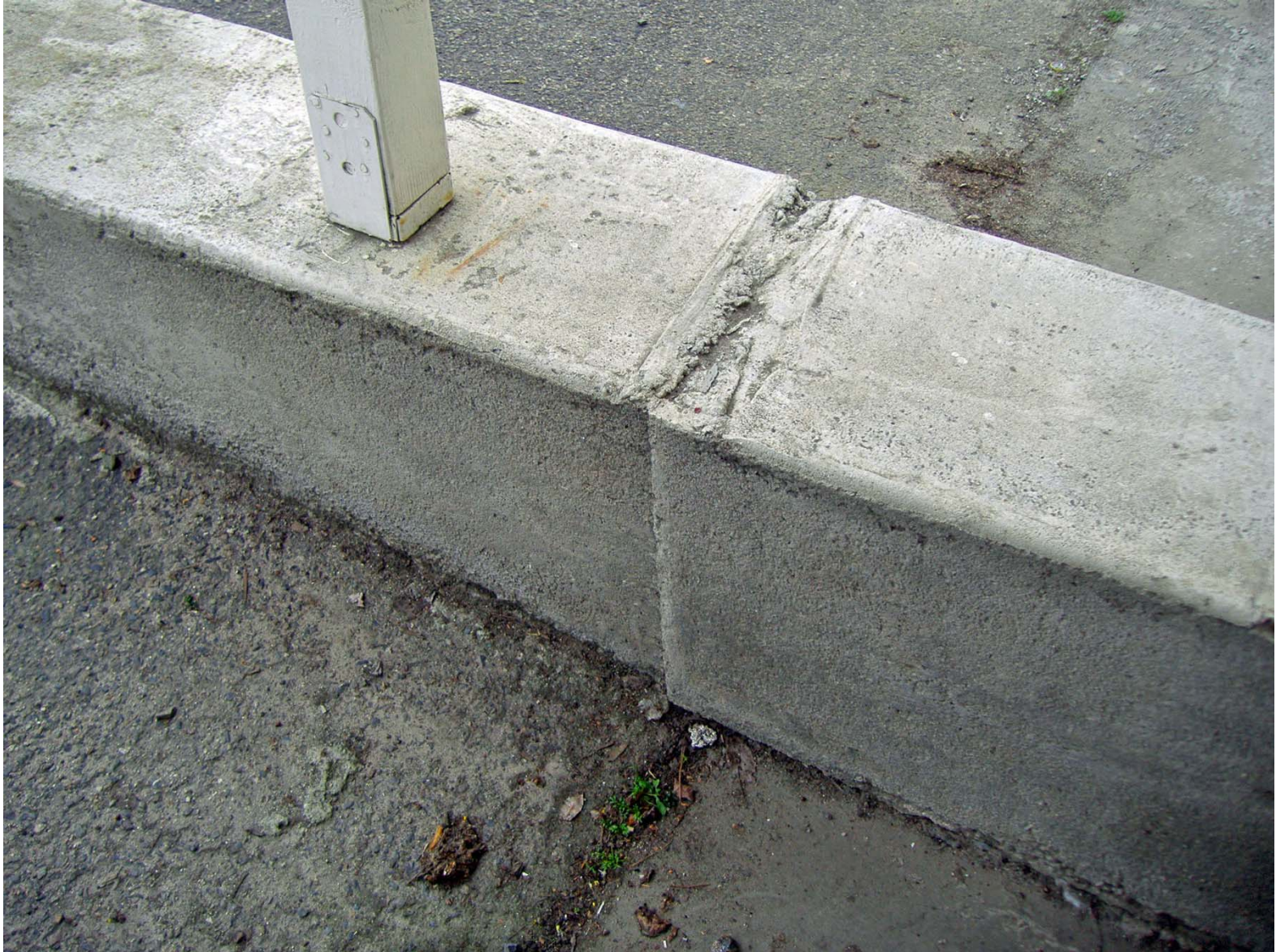
Seam in Concrete Illustrating Additional Concrete Sill Development.
